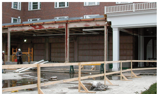
The new Visual Arts Center is set to open in November 2012, while the Hanover Inn's lobby has been temporarily cleared out during renovations.
